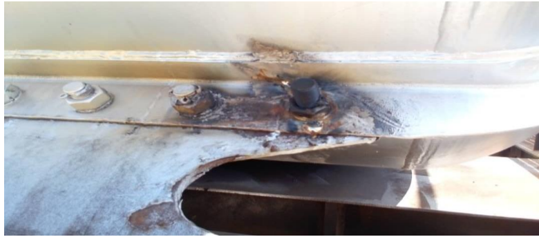
Figure 3.7 Failure zone in the extreme screw hole after repaired. Source: (Author).
